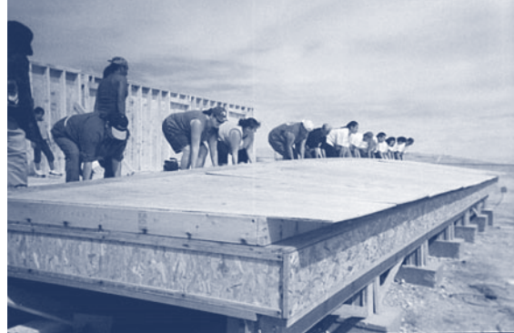
Families work in groups to construct their homes through the Oglala Sioux Tribe Partnership for Housing self-help program. Many people from the seven families in Cindy and Bobby Martin-Laiwa's group helped raise their home's walls.
