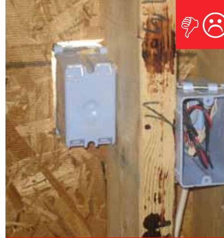
B. Electrical box not air sealed.
