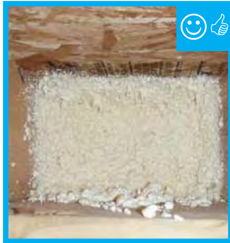
Air barrier is present and installed between the floor system and unconditioned space.
