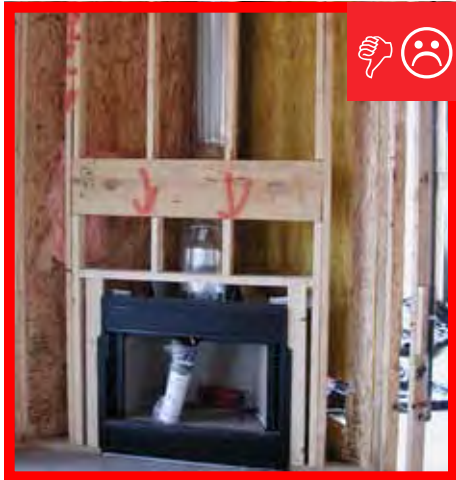
A. No insulation installed behind fireplace.
