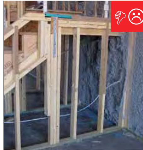
B. No air barrier installed under staircase.
