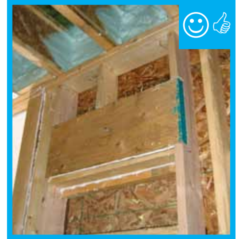
D. Verify single member headers with insulation on one side are installed.
