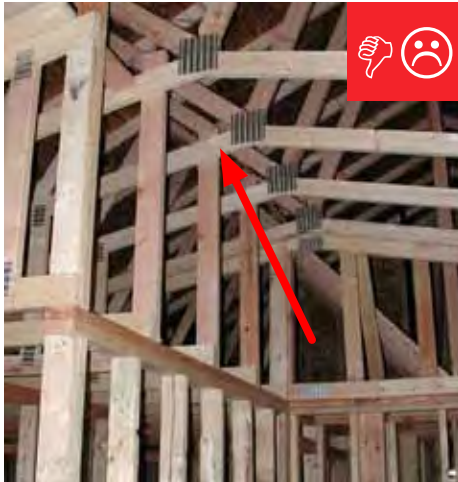
A. No top plate installed.
