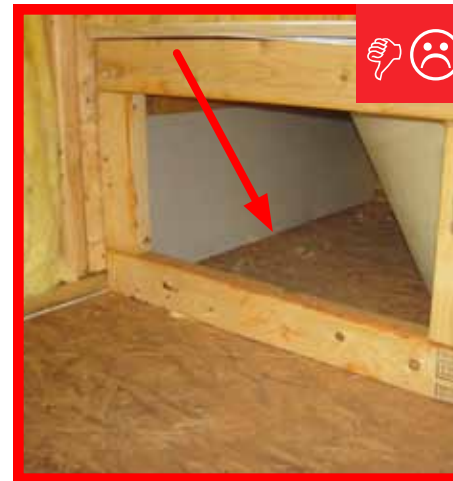
C. Air barrier not sealed.
