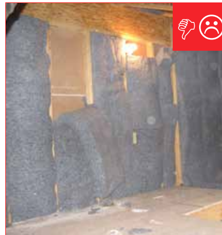
E. Improperly installed insulation and no rigid backing.
