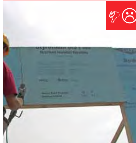
B. Rigid insulation is being installed without cap nails.
