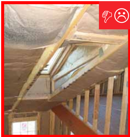
C. Insulation is misaligned with air barrier.
