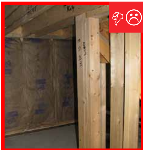
B. No air barrier installed under staircase.
