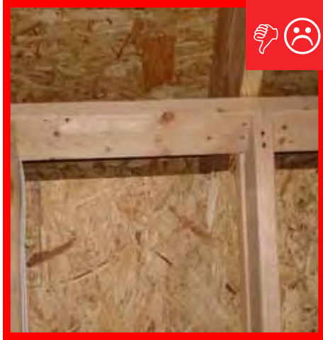
A. Air barrier is not continuous.
