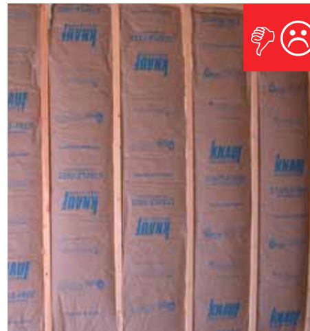
C. Insulation is misaligned.
