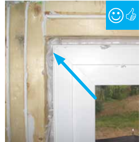
Rough opening around window has been filled with low-expansion foam to air seal.
