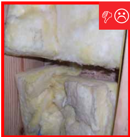
C. Sub-floor insulation has gaps, compression, and misalignment.
