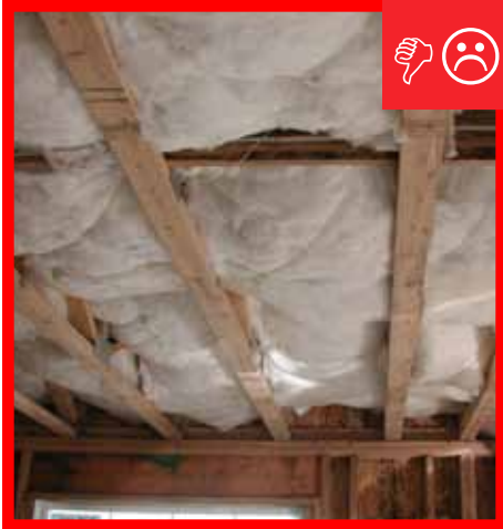
A. Insulation has misalignment, compression, and gaps.
