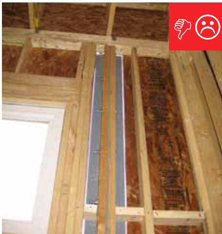
B. Air barrier is air sealed.
