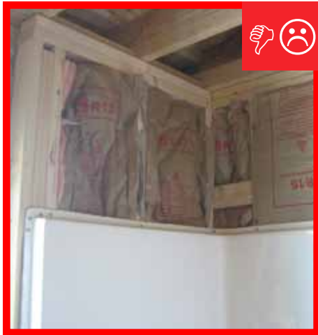
A. Insulation has compression and misalignment.
