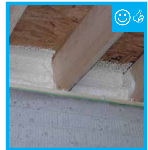
Band is properly insulated and sealed.
