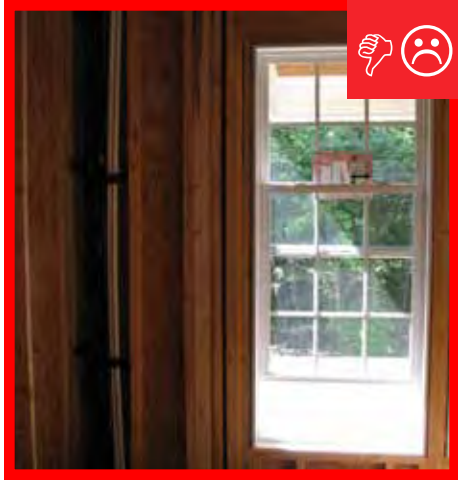
A. Excessive framing and improper spacing of studs.
