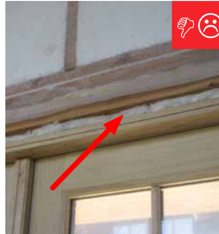
B. Fibrous insulation is not an air barrier and cannot be used to air seal openings.
