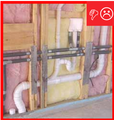
A. Compression and misalignment because insulation is not split around plumbing.
