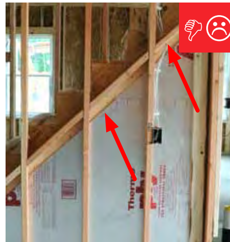
C. Air barrier not sealed.
