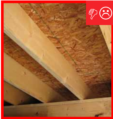
A. No air barrier is present between the floor system and unconditioned space.
