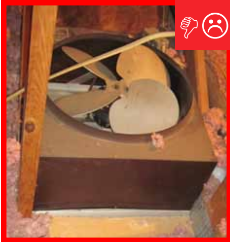
A. Whole house fan installed without an insulated cover.
