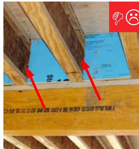
C. Gaps without insulation and not properly sealed.
