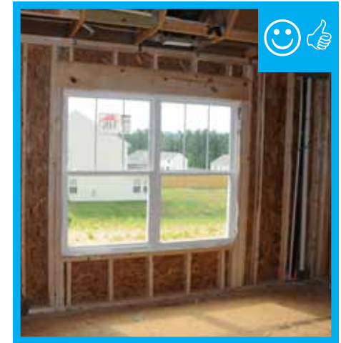
Appropriate use of framing members to support double windows and additional cripples for drywall purposes.
