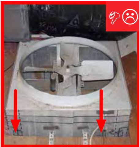
C. Whole house fan installed with holes in surrounding platform that need to be air sealed.
