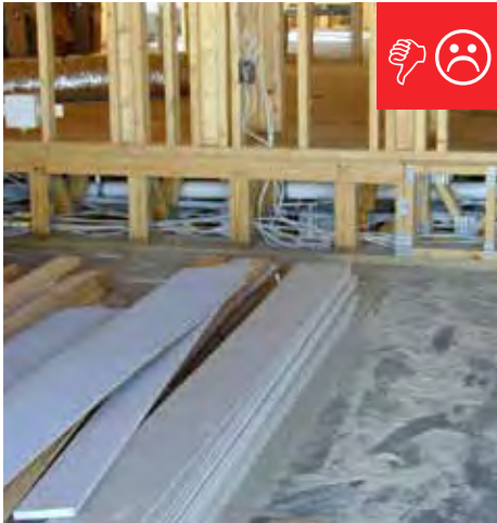
A. No air barrier is present between garage and floor system.
