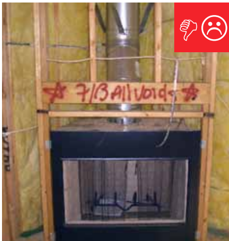
B. No rigid air barrier is installed behind fireplace.
