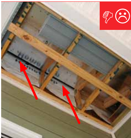
B. Air barrier not sealed between porch attic and conditioned space.
