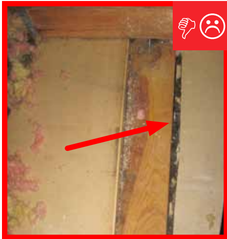
A. Top plate to drywall connection not sealed.
