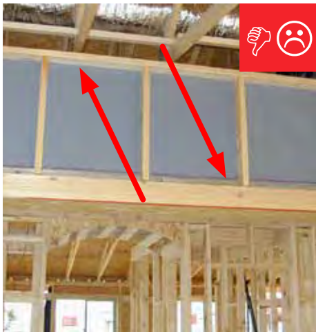
D. Backing not air sealed prior to insulation.
