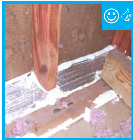
Blocking installed and air sealed instead of continuous top plate.
