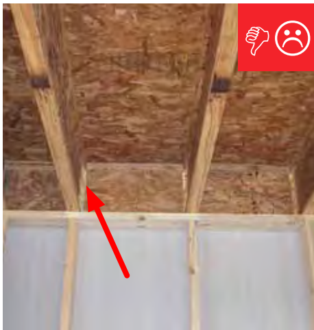
B. Band not properly sealed.
