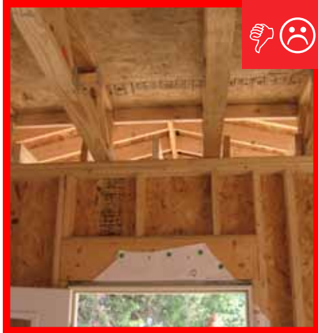
A. No air barrier between porch attic and conditioned space.
