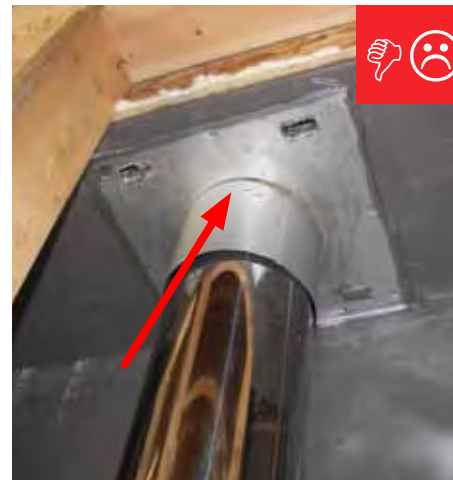
C. Vent sleeve not completely sealed.
