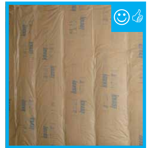
Insulation is properly installed.
