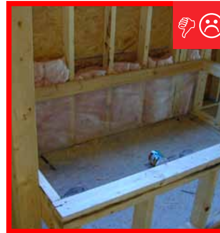
B. No air barrier installed prior to tub installation.
