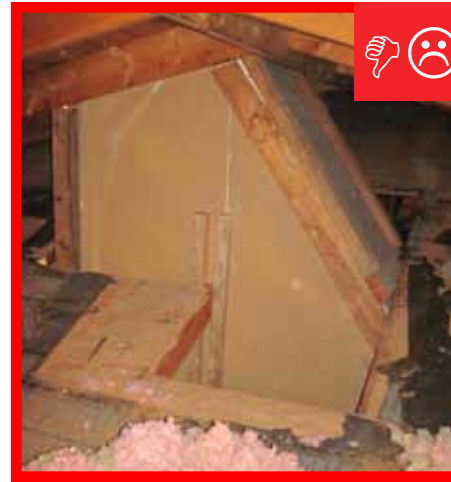
B. Rigid air barrier not properly sealed around skylight shaft.
