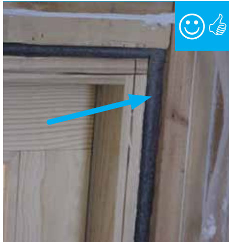
Rough opening around window has been filled with backer-rod to air seal.
