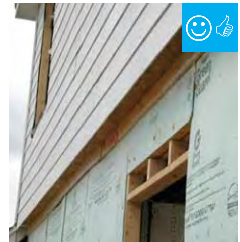
Cantilever has been properly insulated, air sealed, and cavity has been blocked.
