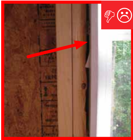
A. Rough opening around window not air sealed
