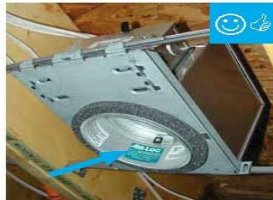
ICAT labeled recessed light with trim kit installed.
