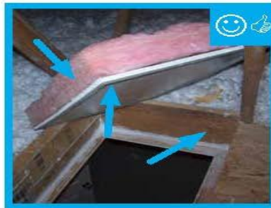
Attic access hatch has been properly insulated by attaching a fiberglass batt, gasketed, and opening has blocking.
