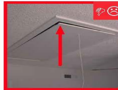
C./D. There is no weather stripping or gasket around the attic stair hatch.
