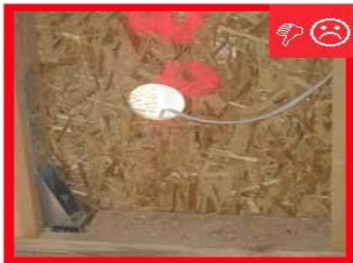
A. Holes have been cut excessively larger than needed making it difficult to seal.
