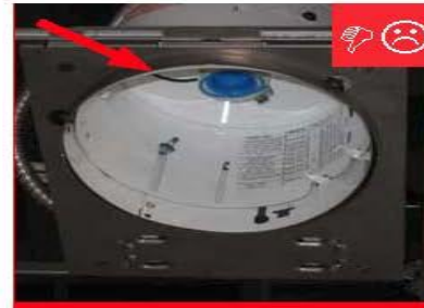
C. No gasket installed.
