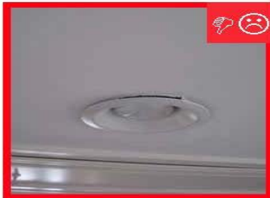
B. Recessed can light has not been sealed to drywall.
