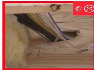
A. Hole was not neatly cut with a saw making it difficult to seal.
