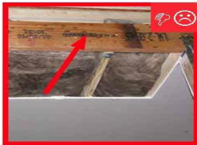
A. No gasket installed at marriage wall connection prior to assembly.
