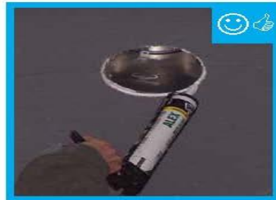
Recessed can light penetration sealed with caulk to drywall.
