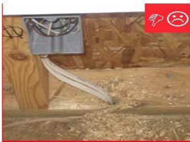
B. Hole has not been air sealed.
