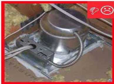
A. Non ICAT recessed light installed.
