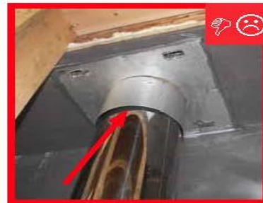
D. Vent sleeve not completely sealed.
