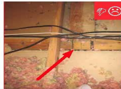
A. Top plate to drywall connection not sealed.
