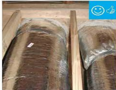
Chase capped with rigid air barrier and duct work penetrations properly sealed.
