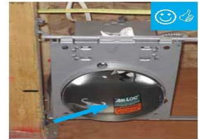
ICAT labeled recessed light installed but still needs gasket.
