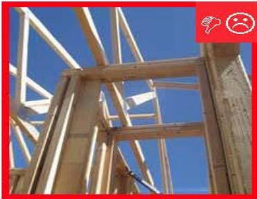
A. Chase not capped.
