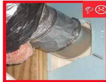
B. Penetration hole is larger than duct and not sealed.
