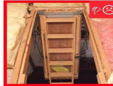
B. Drop down stairs do not have an insulation cover installed.
