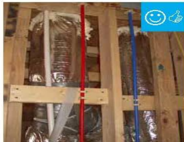
Penetrations have been neatly cut and properly sealed with foam.
