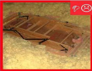
A. No blocking installed to prevent attic insulation from falling into stairs and opening.
