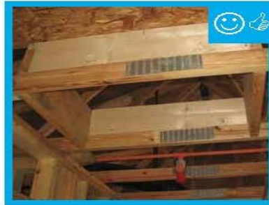
Blocking has been installed around the perimeter of this attic access to prevent insulation falling into the house.
