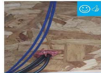
Wiring penetrations have been neatly sealed with foam.
