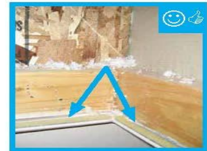
From inside attic: this attic access door has a foam and rubber weather-stripping installed that remains in contact when closed.
