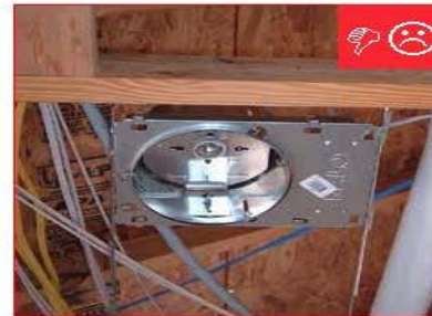
A. Non ICAT recessed light installed.
