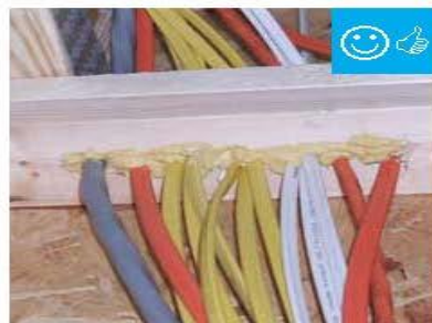
Wiring penetrations have been neatly sealed with foam.
