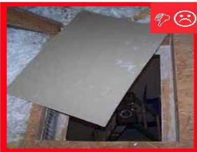
B. Attic access panel does not have an insulation cover installed.
