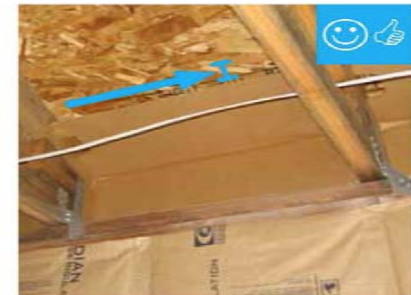
Wind baffle installation maintains necessary code clearance between baffle and roof deck.
