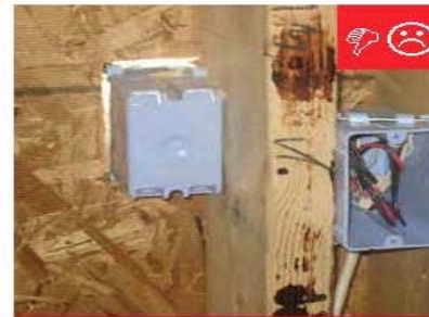
B. Electrical box not air sealed.
