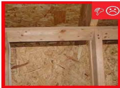
A. Air barrier is not continuous.
