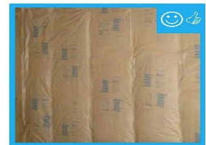
Insulation is properly installed.
