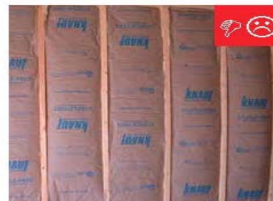
C. Insulation is misaligned.
