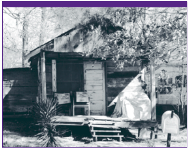
Lack of an adequate supply of affordable housing forces many low-income families in West Feliciana to live in substandard housing such as this dilapidated unit.
