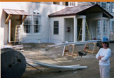
Windham Housing Trust (formerly Brattleboro Area CLT) is a recipient of assistance under HAC's Rural Community Development Initiative that is converting an old warehouse into affordable rental housing and office space. Pictured is Connie Snow, Executive Director of WHT.
