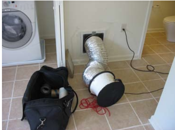
A duct-blaster test pressurizes the duct system to measure the air-tightness of the system.
